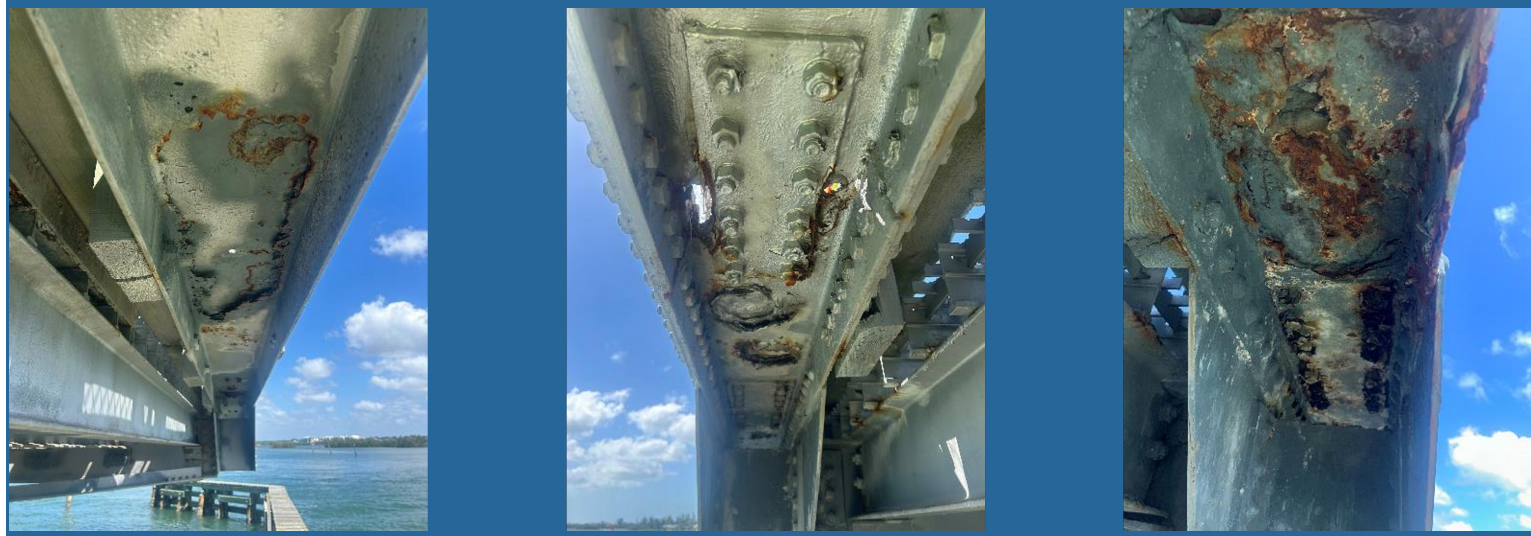
These images show active corrosion on structural components of the bridge.
